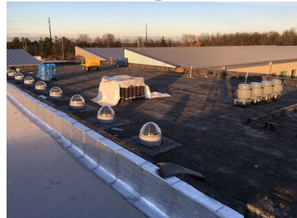
Roof Showing Solatubes
